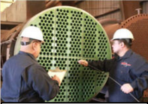
MICRO BLASTING & NANO COATING
